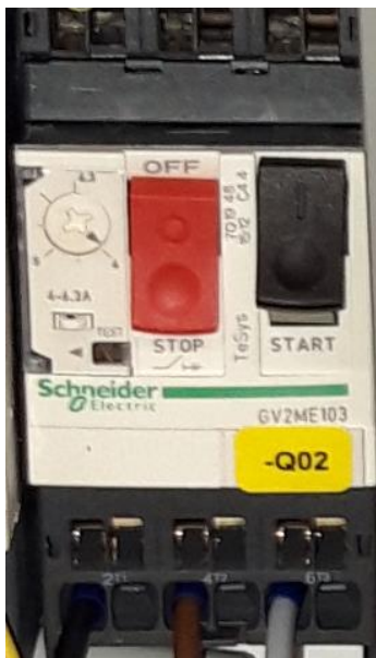
Figure 29: Circuit breaker with overcurrent protection
