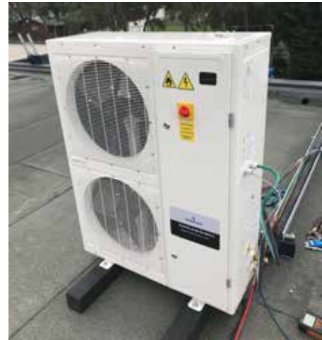
Copeland ZX A2L refrigeration unit, installed at Delhaize supermarket, in Belgium.
