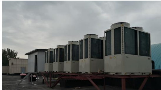
R32 heating project in a shopping mall in Yining, Xinjiang
