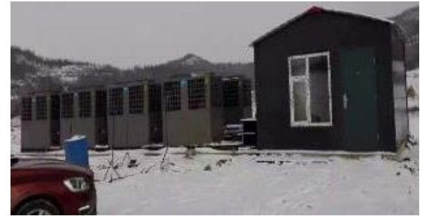
Heat pump heating project of a ski resort in Jilin
