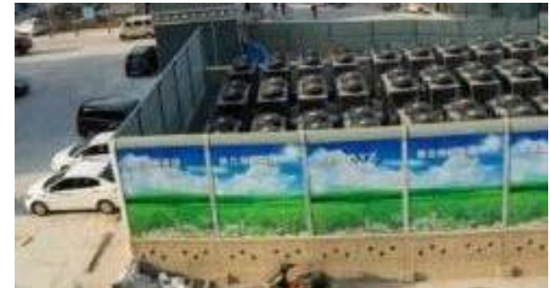
District heating project of a community in Shandong
